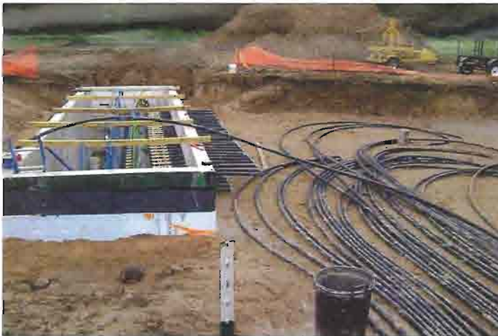
The concrete vault, now underground, houses the piping manifolds.
