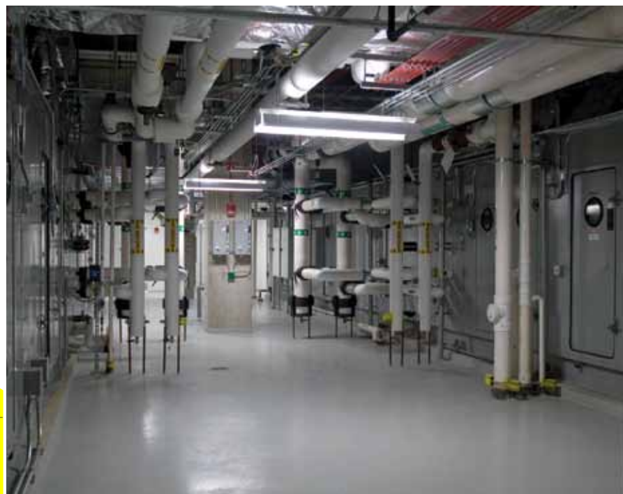
The mechanical room at Columbia St. Mary's Hospital, Milwaukee.
