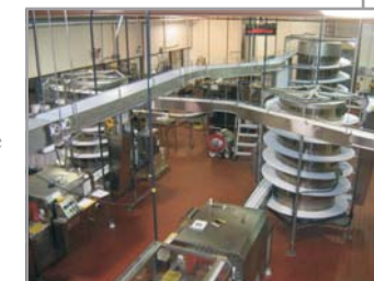
HiMEC installed spirals and conveyor systems in the Kemps Packaging Room.
