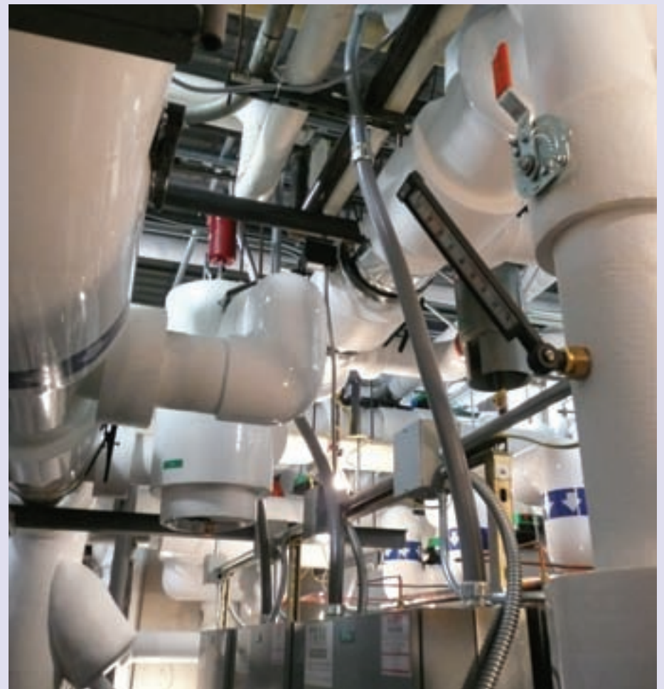
Piping connects to the heart of the GeoExchange system.
